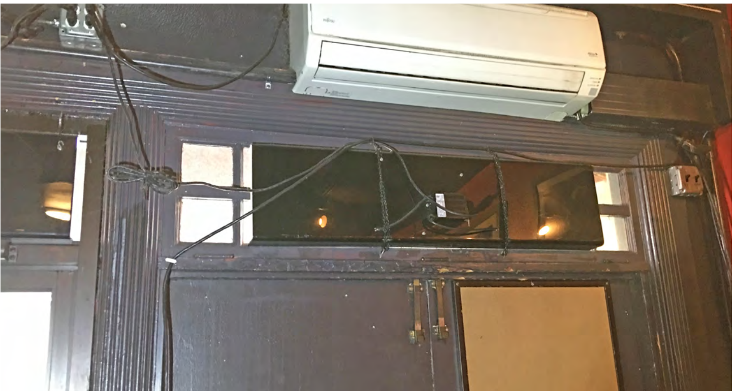
Figure 21. Showbox, detail view of the interior face of the doors showing the reeded detailing original to the 1939 remodel that is replicated on the exterior side of the doorways as well. The wood sash transom is also visible.
