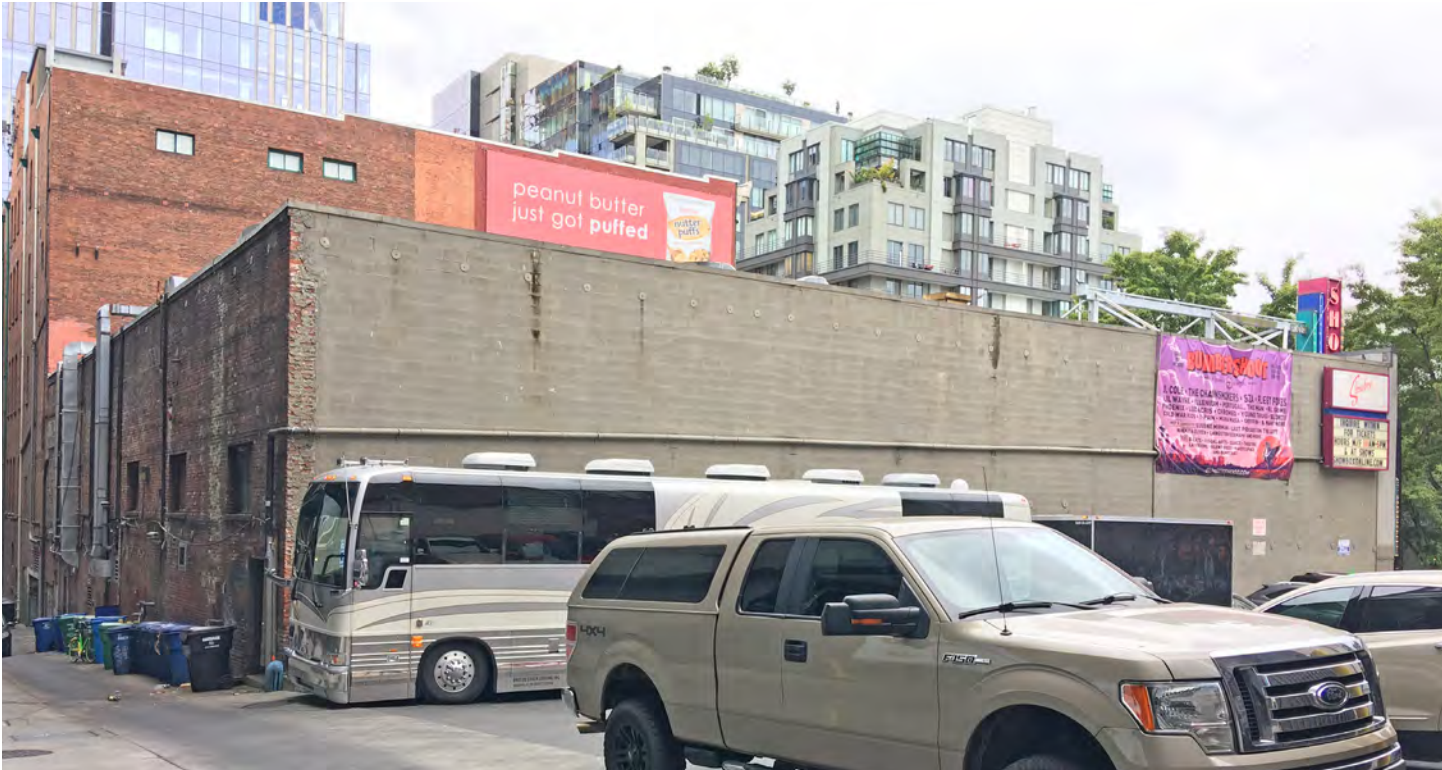
Figure 13. Northeast corner, looking southwest along the alley. The reconstructed north wall is visible.
