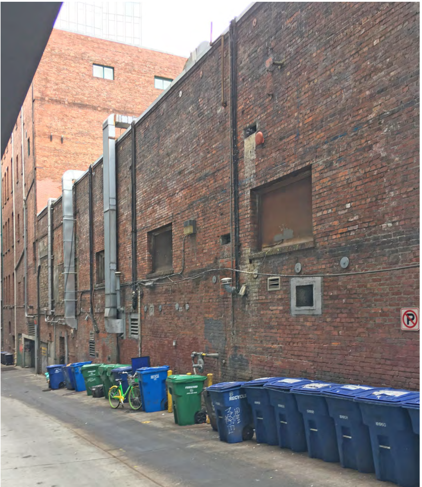
Figure 14. East alley facade looking south. The load bearing brick construction stems from the building's 1916 construction.
