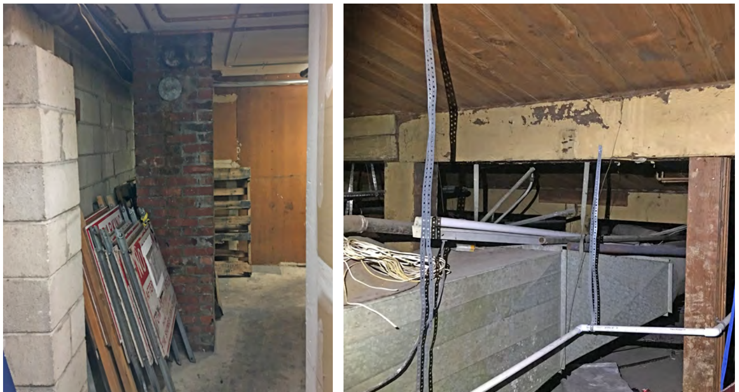
Figure 52. Service area, looking east along the rebuilt north facade. The brick chimney is original to the 1916 construction of the building (above left). A view looking west (above right) below the Showbox passageway showing the framing and ramp that are original to the 1939 remodel.
