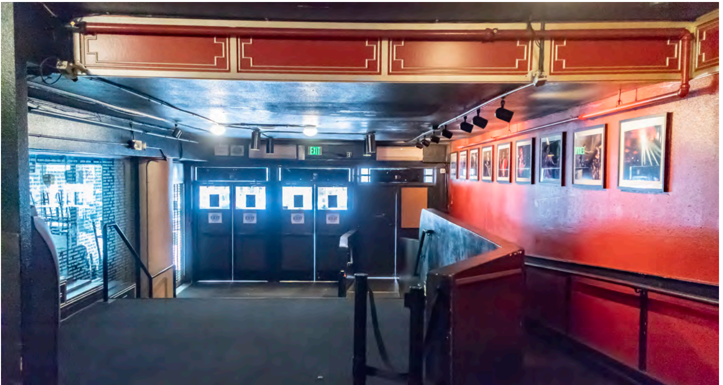
Figure 20. Showbox, looking west along the passageway at the three doorways providing access. The soffit above marks the line of the second floor framing. The volume of this passageway, door surrounds, and the large column at left are original to the 1939 remodel creating the Showbox.
