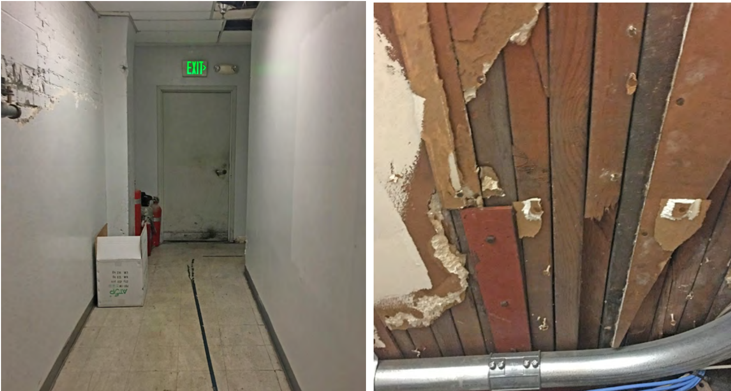
Figure 53. Service area, looking east and showing typical wall finishes (above left). The wall along the left side is the outer brick masonry wall. Note the brick pier that steps out to support the massive east to west beams carrying the second floor. A detail (above right) of the crib construction (2x boards on edge) comprising the floor structure for the second floor.
